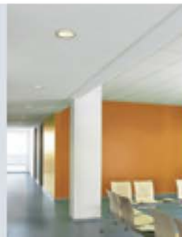
Fire protection ceilings
